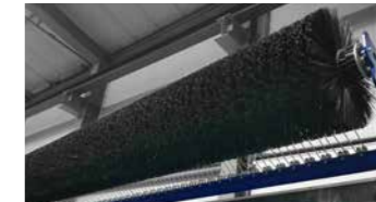
Brush cleaning springs
