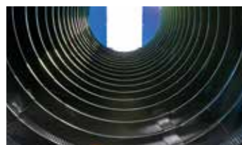
Screw conveyor internal
