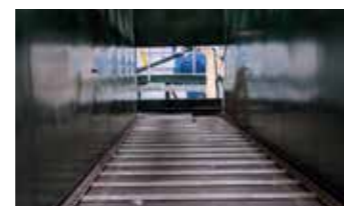
Bunker with scraper chain conveyor
